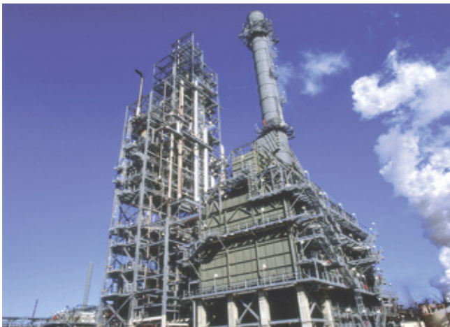
Photo of Catalytic Reformer courtesy of CB&I
