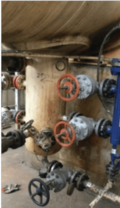
Refinery unit with boot as liquid-liquid separator
