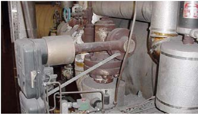
Modernizing feedwater heater level controls allows operators to better manage controllable losses while significantly reducing maintenance costs. Torque tube displacers (above) are common in the industry and one of the easiest to retrofit.
