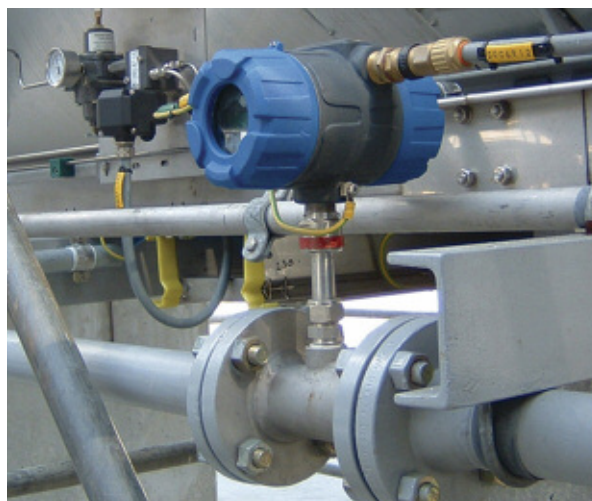
Measuring natural gas flow to a furnace. The use of an insertion probe permits the TA2 to be installed in lines of various sizes and with considerable installation flexibility while also ensuring economical mass flow measurement.
